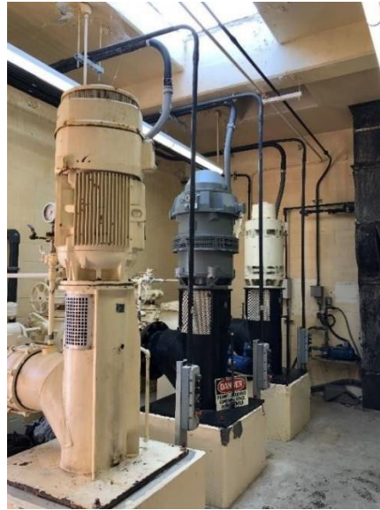
Effluent pumps 1, 2, and 3
